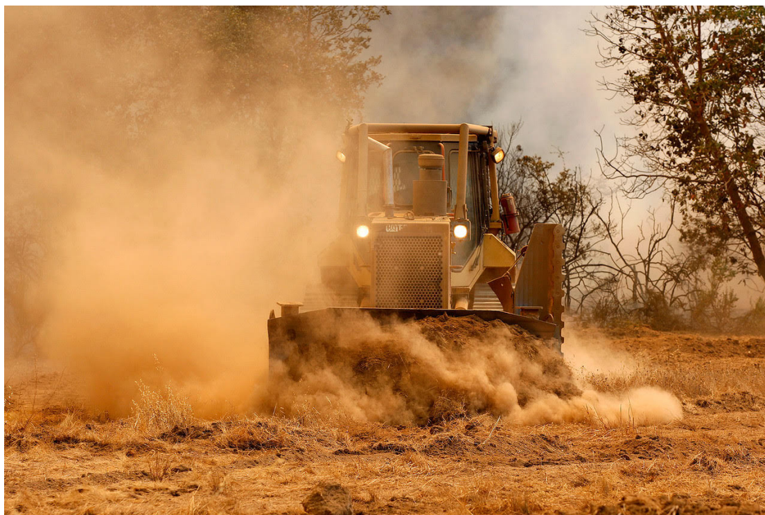
Image 10: A bulldozer cutting an indirect fireline on the Soberanes Fire. Over 20 miles of dozerlines were carved into the Ventana Wilderness Area. Image courtesy of USFS.
